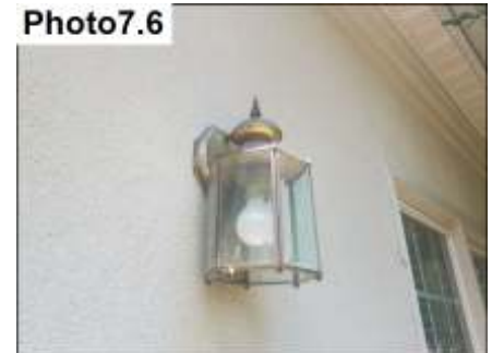
All lights need caulking.
