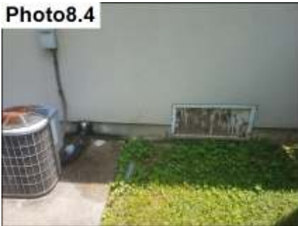
Crawlspace door needs to be caulked.
