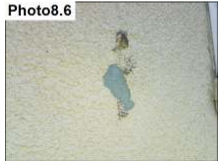
Finish need to be added to this chipped area.(G5)
