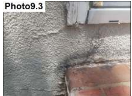
Area below door is delaminated and needs repair.
