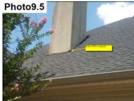
Bottom of chimney needs repair.
