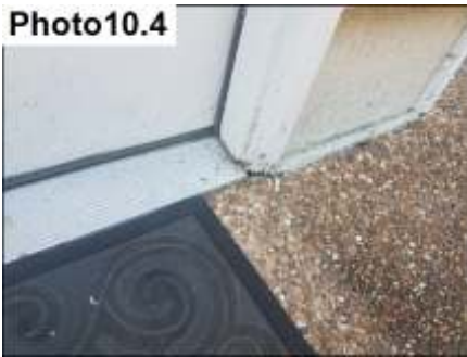
Brick mold at bottom of door needs replacing.
