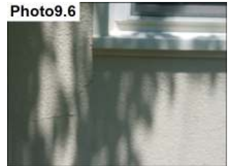
Bottoms of these door are rotting.
