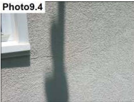
Small Crack at J5.
