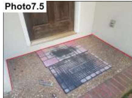
Porch needs caulking, theshold needs caulking and electrical socket
