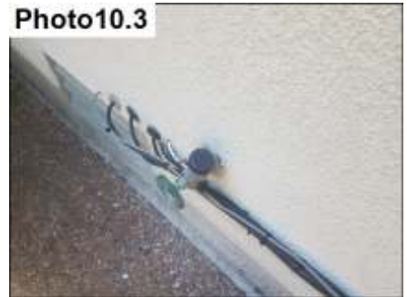
Hose bibbs need caulking.
