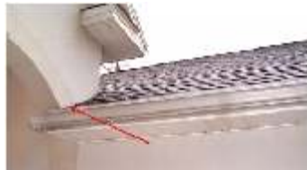
Figure 1: No kickout flashing
