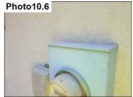
Utility boxes need caulking.
