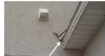
Fig 2: Improper installation (unsealed)
