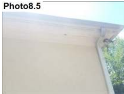
Bird hole needs to be repaired.(J4)
